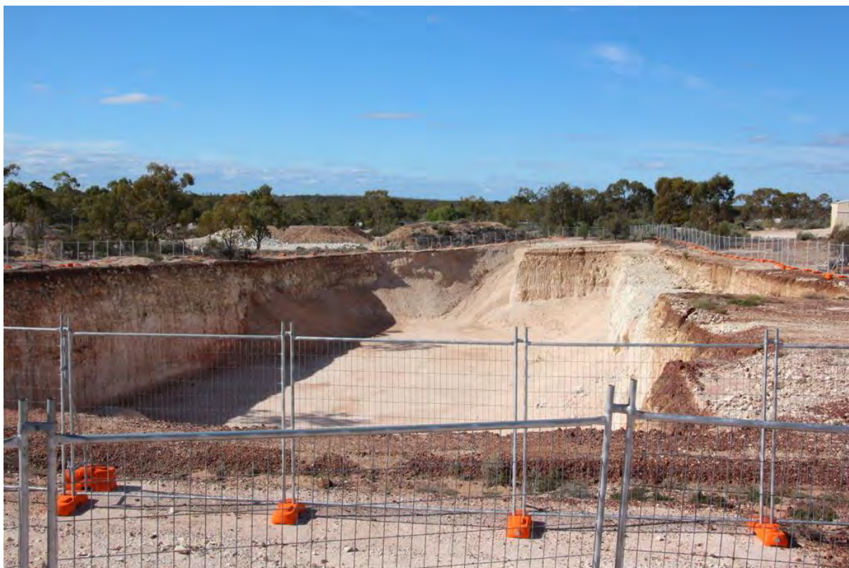
Large hole in the ground – site of the future Australian Opal Centre. Photographer: Gerry Kool.
